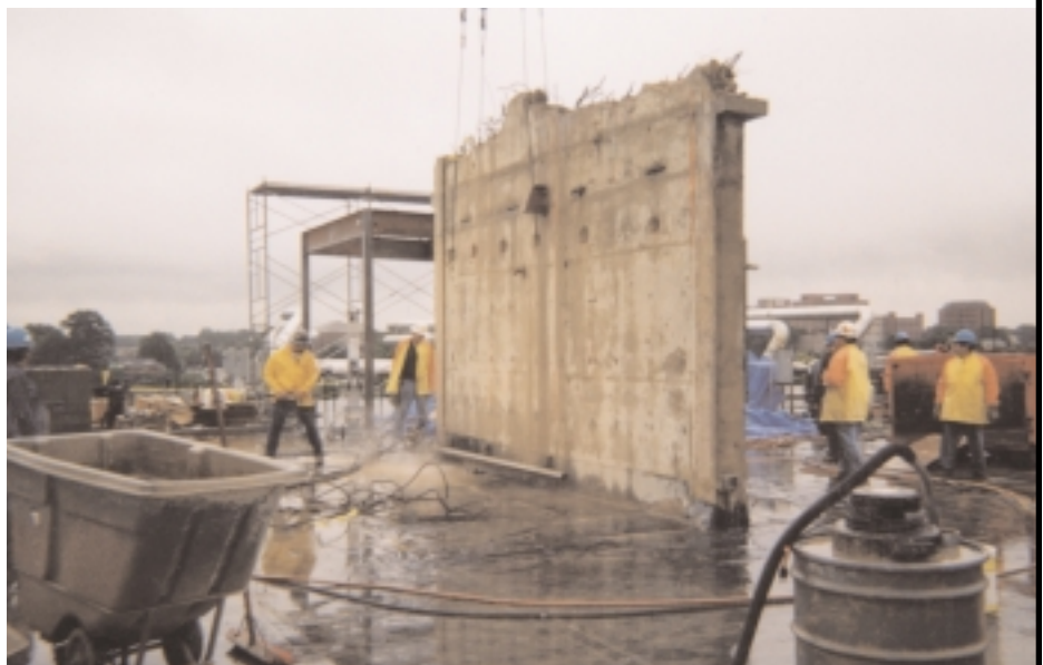
Above Top: The first step was to remove the cantilevered floor to be able to gain access to the concrete panels underneath.
